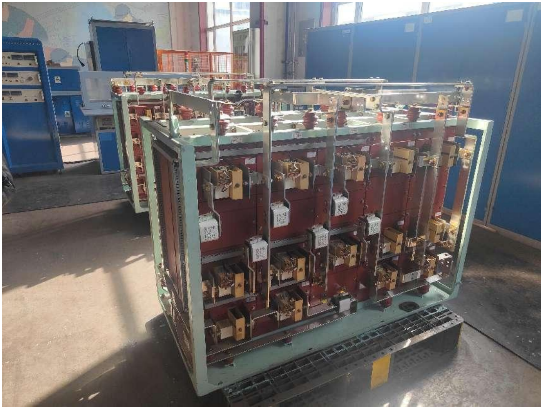
Figure 6 Physical photo of SS3B rectifier cabinet
